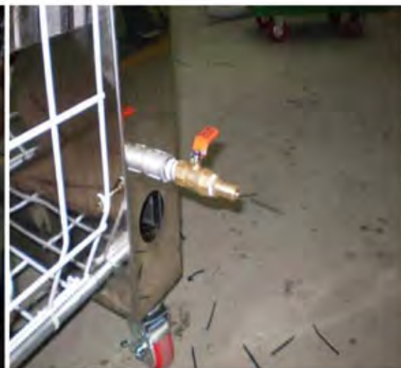
WATER SUPPLY VALVE
